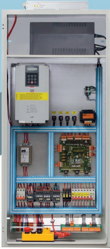
HIZ KONTROLLÜ KURTARANLI PANO VVVF CONTROL PANEL
